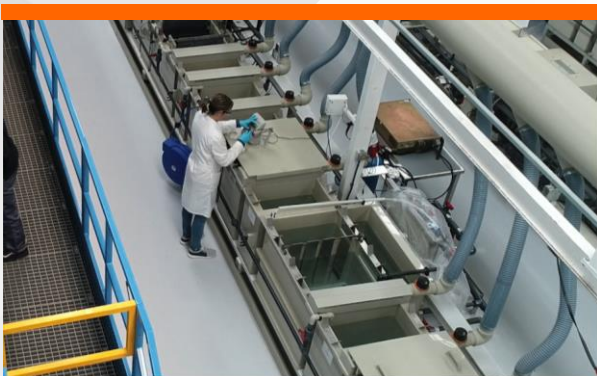
ANODIZING AND E-COATING MODULE
